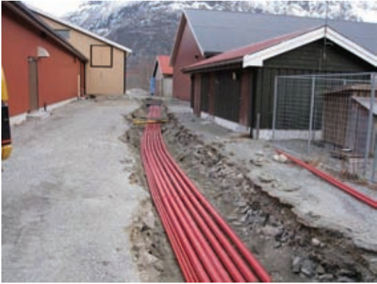
Cabling is laid for electricity, data and telecommunications along with the pipework for the cooling system.
