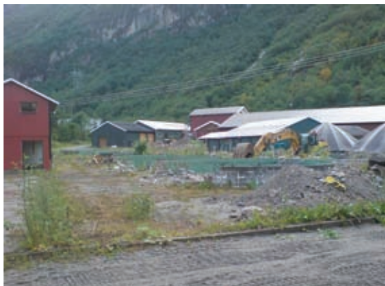
The site before building began. The old 11 m ponds will be removed.
