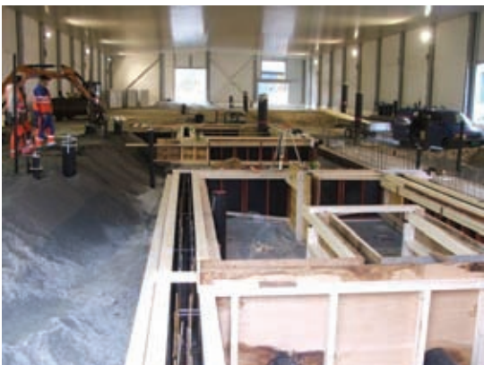
A sunken area is framed in, there is a 12 m 3 /min pump sump visible in the foreground.
